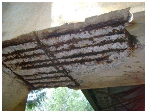
Figure 1.2: Corrosion of steel reinforcement due to de-icing salts in a parking garage 2 .
