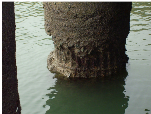
Figure 1.1: Rebar corrosion in a concrete pile in a marine structure in the splash and tidal zones 1 .
